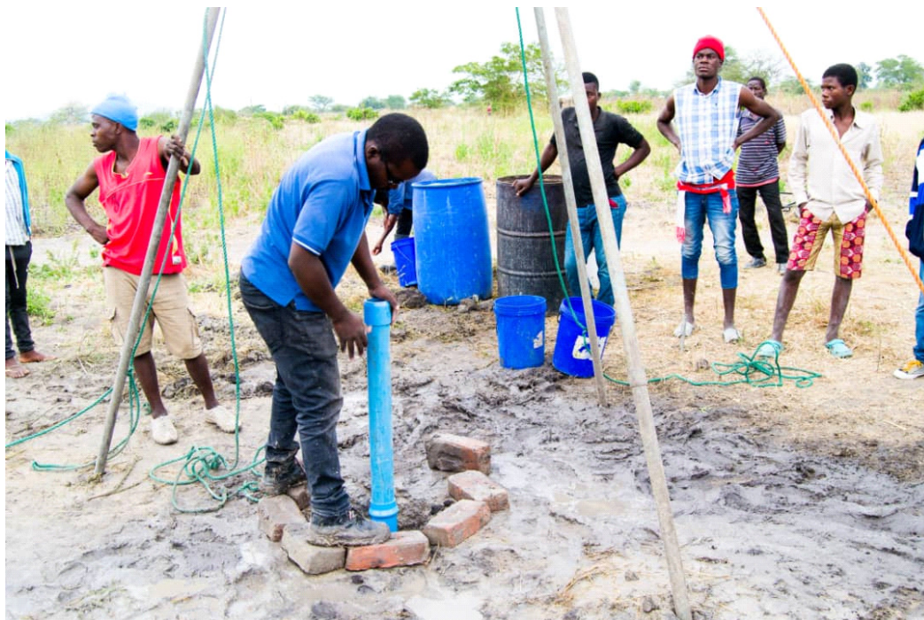
George Mkoko, country coordinator, inspecting installation of 90mm liner prior to pump installation
