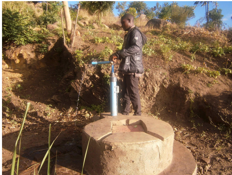
One of the two pump installations sponsored by the donor family
