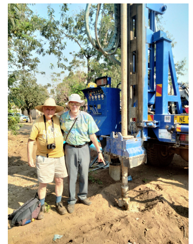
Mike of Seedsowers with Matt of Hope in Africa witnessing the drilling of the borehole at Nsanje
