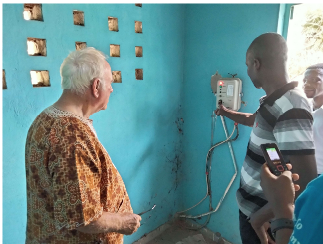
Seedsowers's Chairman being shown the controls for the newly installed Solar Pump which pumps water to the Lundu Health Centre
