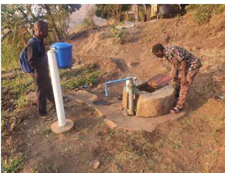
The second damaged RORA donated borehole before refurbishment
