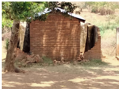
Girls toilet before refurbishment
